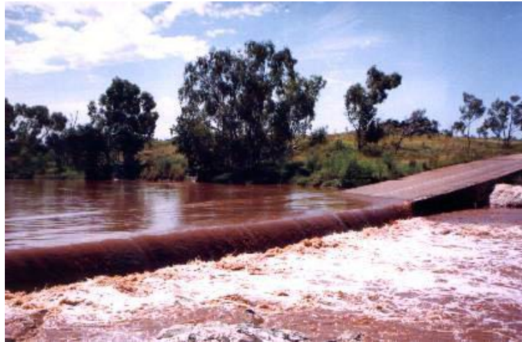
Little Panton River flooding Highway One
